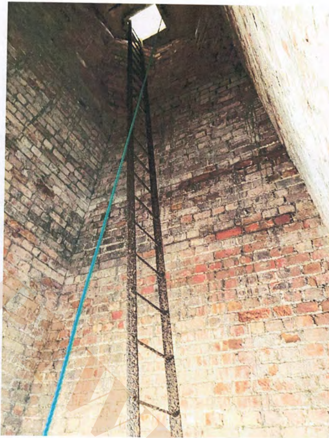
12.4 Tower lower chamber ladder
