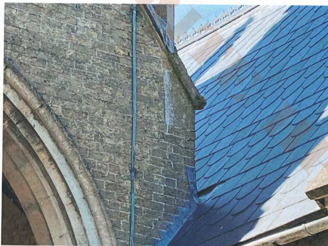
8.5 East elevation cracking 8.7 kneeler
