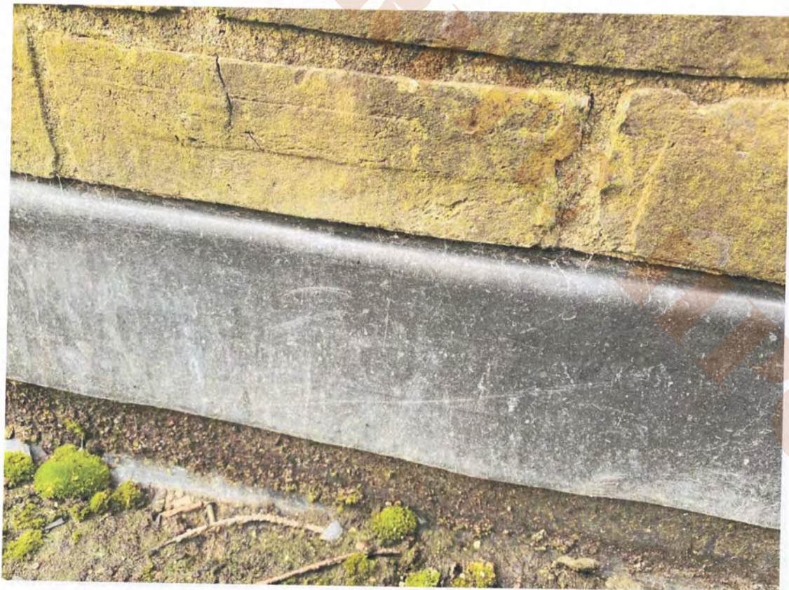
7.12 North chapel south roof/ tower flashing
